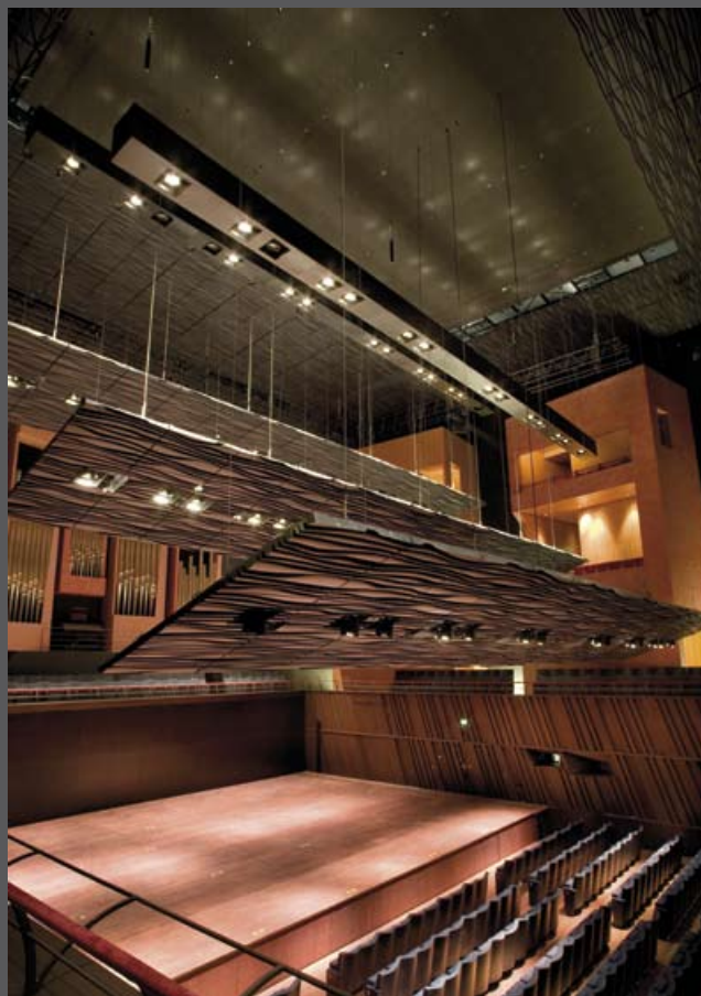
Powerful and silent! Floating lighting, hung from the ceiling of a philharmonic.
